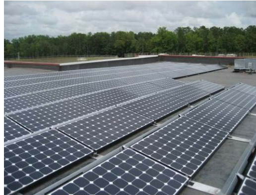
Figure 1: T-10 system on roof of LCJC
