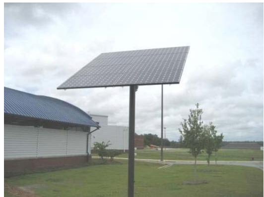
Figure 2: Pole mounted array at LCJC
